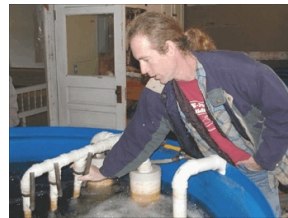
John Stewart adjusts the nozzles on the filter and circulation unit at Aquaculture Engineering USA.
